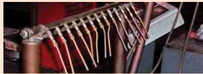
Turbulent compressed air blasts straight out of the pipe or tube. It not only wastes huge amounts of compressed air but also violates OSHA noise and dead end pressure requirements.
