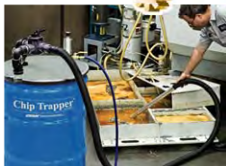
Chips can accumulate in the sump, restricting coolant flow.
